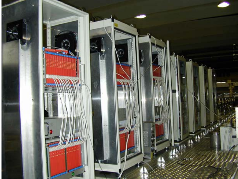
Figure 2: Top side of the T600 module during installation of the electronics racks.
