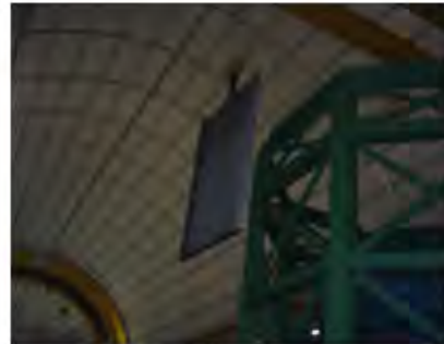
Figure 8: positioning of the first stainless steel box inside the WarP mechanical structure (October 08).
